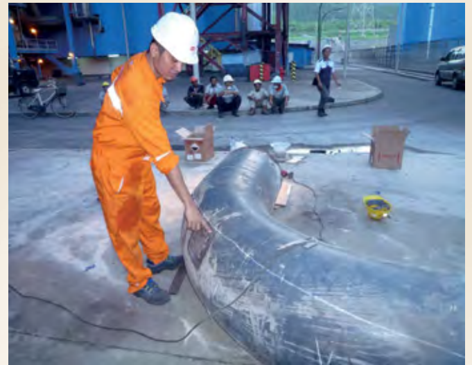
The previous method used was patching from the outside.
